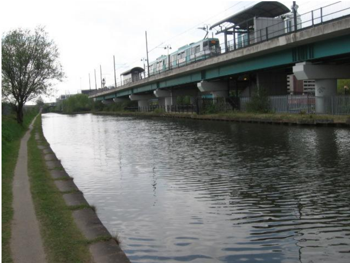
An elevated section of the Phase 2 Metrolink alignment at Pomona – showing the major structures which added to the scheme cost
